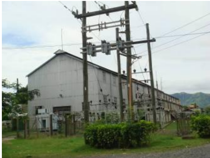
Diesel Power Generation Station
