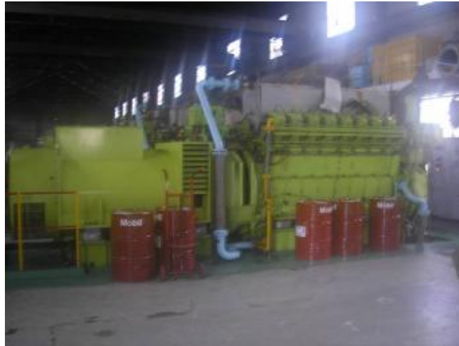
Power house – No 1 Generator set
