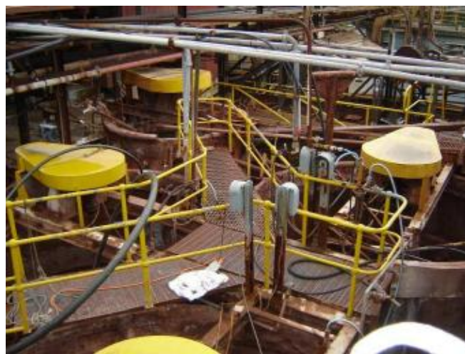
Calcine leach tanks
