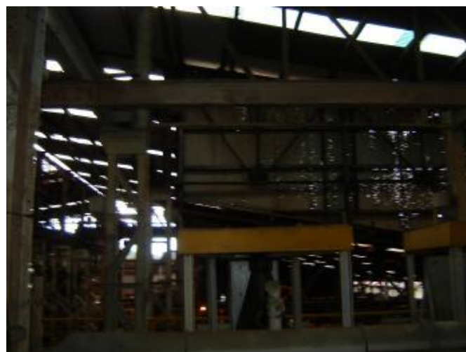
Main flotation plant side panel defects
