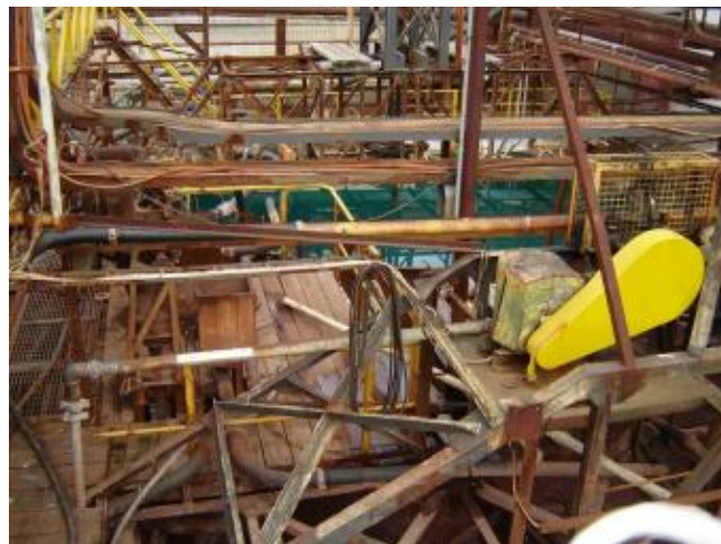
Calcine decant thickener
