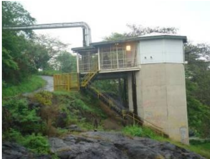
Nasivi River Pump Station
